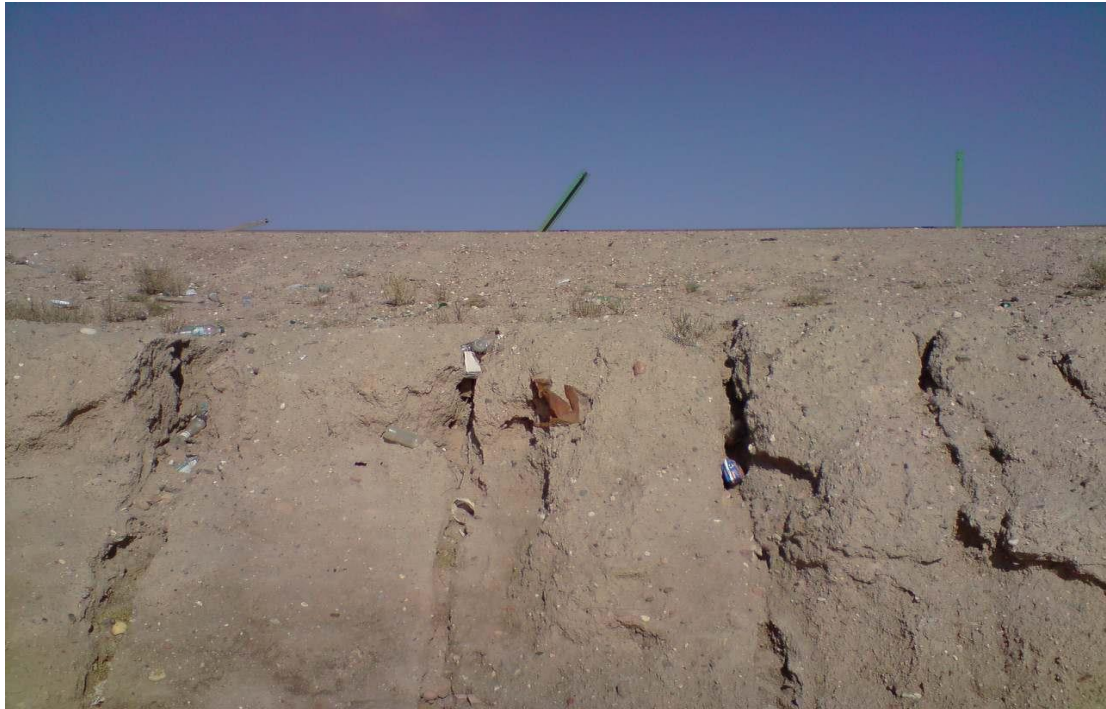
Fig.(4) Study embankment with remarked gully erosion
