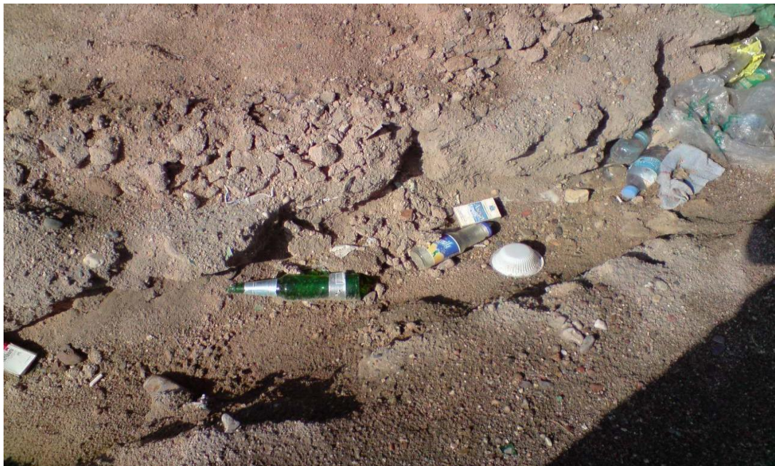
Fig.(3) Study embankment with remarked gully erosion
