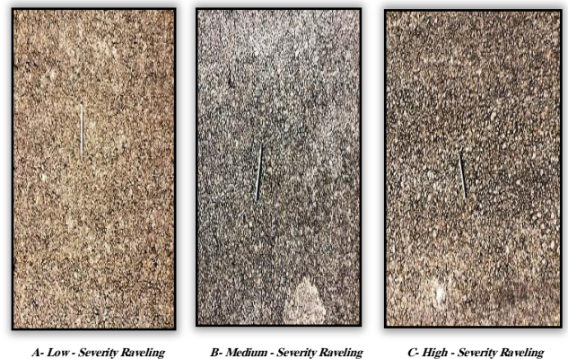
Figure 7. Raveling Distress severity Road No. (3) (Poor condition)
