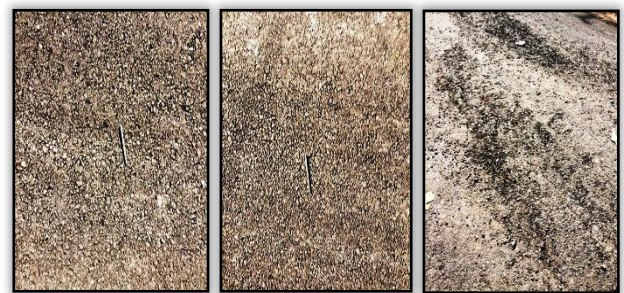
A - Low - Severity Raveling B - Medium - Severity Raveling C - High - Severity Raveling
