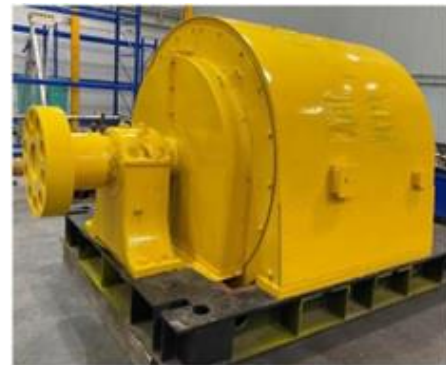
Fig.1 2.5 MW 6.6 kV synchronous motor
