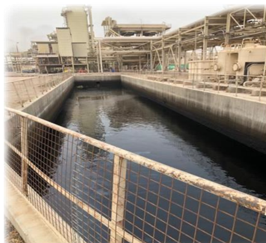
Fig.1 Sedimentation tank and pipes in Gas Company
