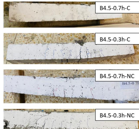
Figure 4: Crack patterns of all beams
